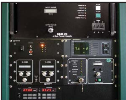
EVAP POWER SUPPLIES & CONTROL
