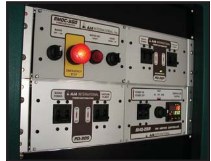
POWER DISTRIBUTION MODULES
